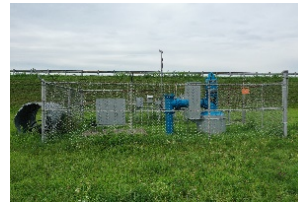
Jacobs supports a variety of project for the Middletown WTP including limes sludge management options and increasing capacity of their system.
