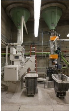
These two lime slakers were replaced with new Chemco slakers for improved maintenance..
